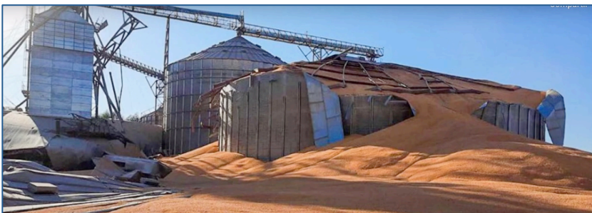
Colapso silo de 15.000 tons (MT), 07/2021
